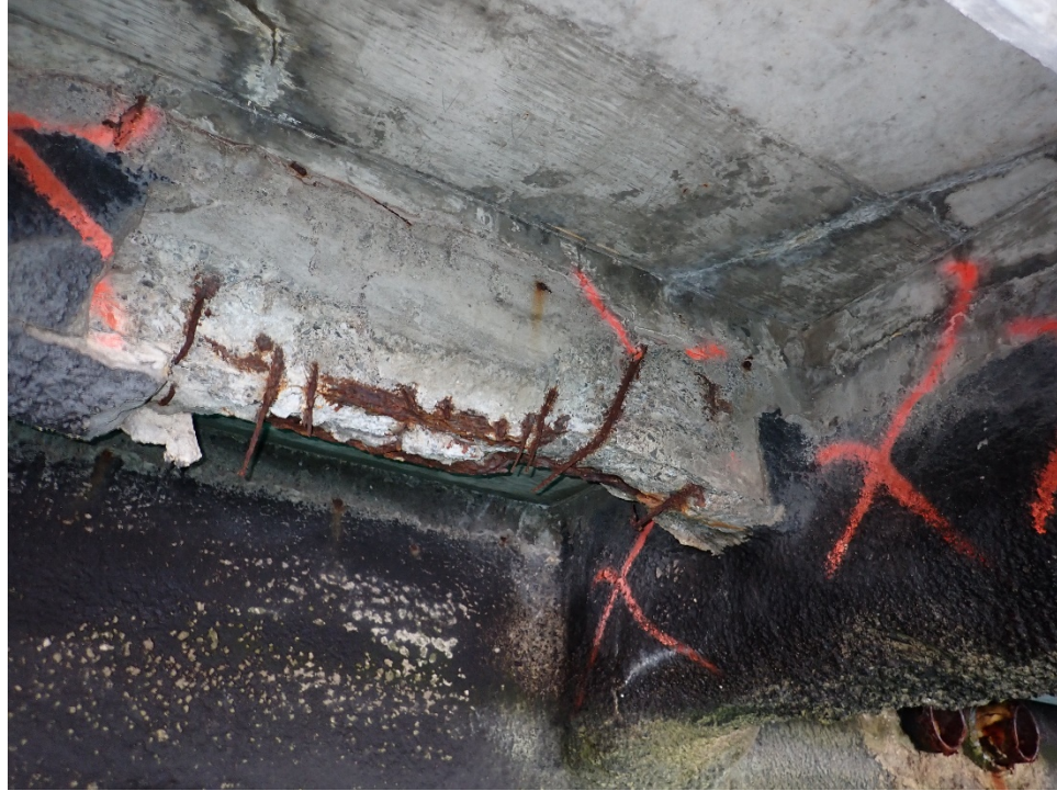
Photo 3: Typical Beam Spall at Pier 10
