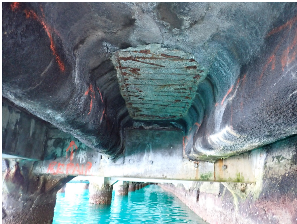
Photo 2: Typical Slab Spall at Pier 10
