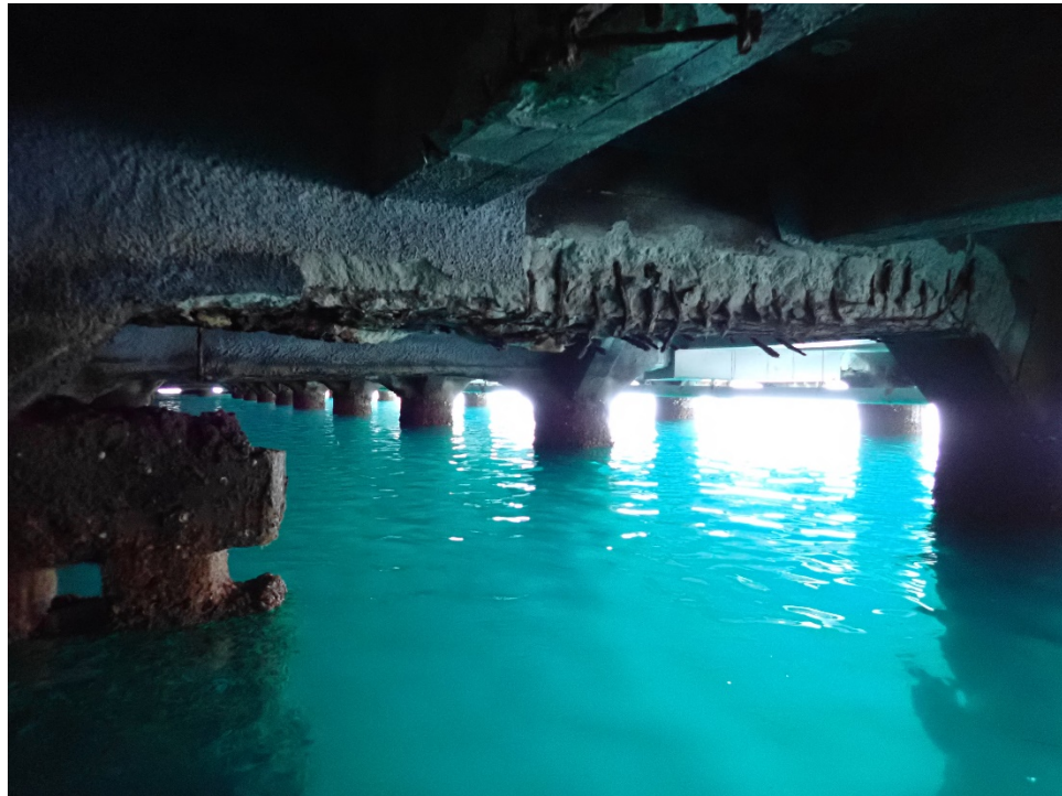
Photo 4: Typical Girder Spall at Pier 10
